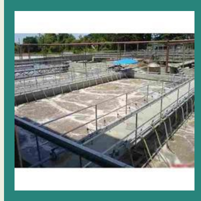
Diffused Aeration System
