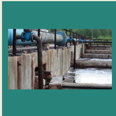
Industrial Sewage Treatment Plant
