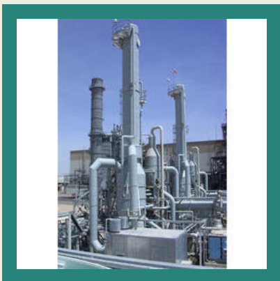
Waste Water Effluent Treatment Plant
