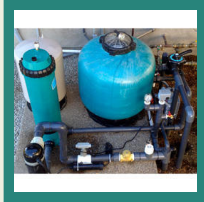
Water Recycling System
