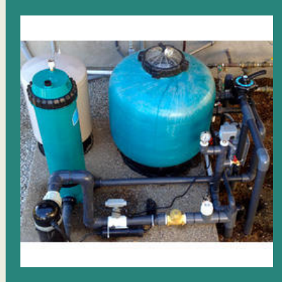
Water Recycling System
