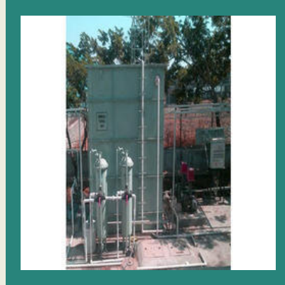
Ready Made Effluent Treatment Plant
