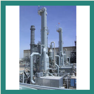
Waste Water Effluent Treatment Plant
