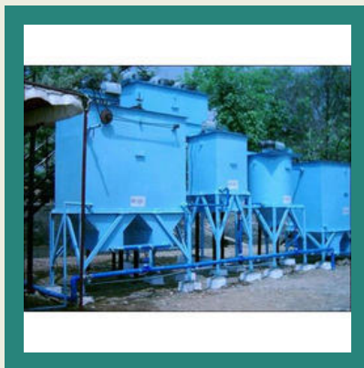
Industrial Effluent Treatment Plant
