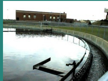
Industrial Water Clarifier Plant
