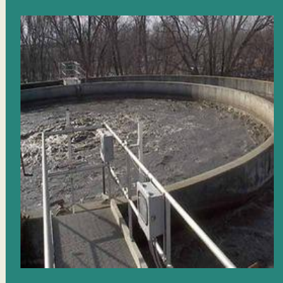
Sewage Water Treatment Plants
