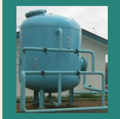
Pressure Sand Filter
