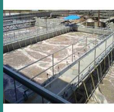
Water Effluent Treatment Plant
