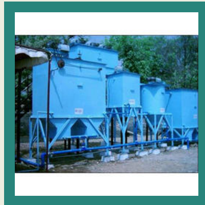
Industrial Effluent Treatment Plant
