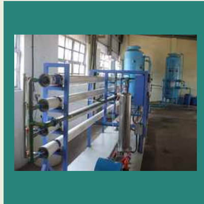
Water Filtration RO System
