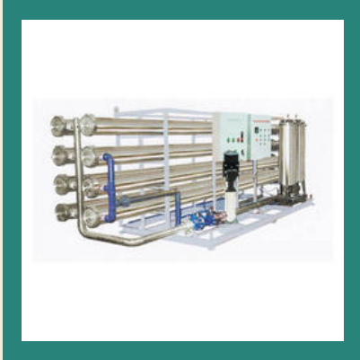
Reverse Osmosis Plant
