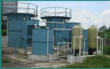
Sewage Treatment Plant
